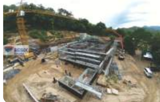
Kumbukkana treatment plant
