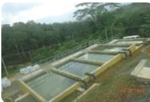
Water Treatment Plant - Balangoda
