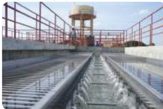
Plate Settlers of Muttur Water Treatment Plant
