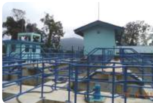
Water Treatment Plant at Ratnapura
