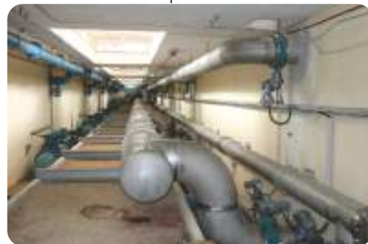
Back wash pumps at Kalatuwawa
